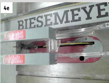
Figure 4e: Table saw blade guard is broken.
